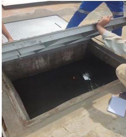
Gambar 10. Unit Biofilter Anaerobik
