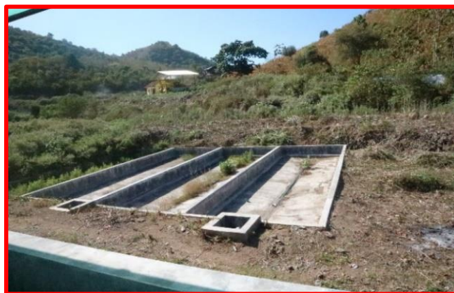
Gambar 6. Sludge Drying Bed (SDB)
